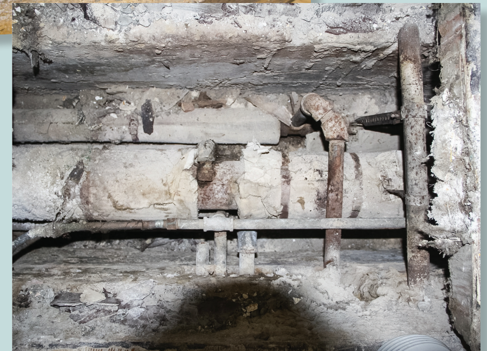
Critical water and HVAC pipes were installed in the perimeter chanel below ground.
