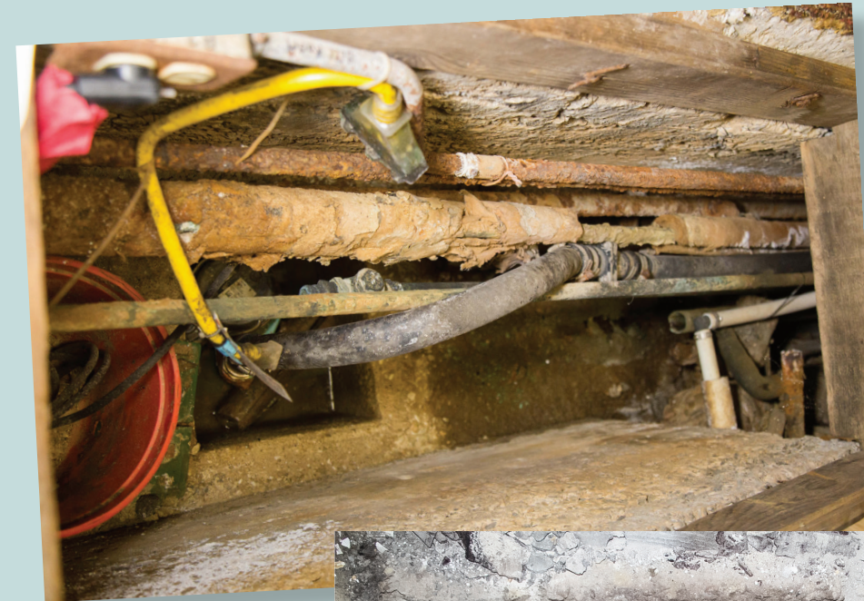
In the southwest entryway men's bathroom, the water pipe corroded and burst, flooding the floor and causing damage to part of the first floor Children's Ministries area, which were removed and replaced.
